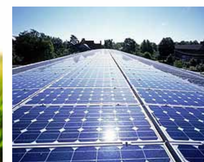
Photovoltaic panels on new roof
